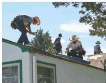
A roofing crew performs repairs in Eads, Colo., where temperatures approached triple digits. Exceptionally hot weather is expected to persist in the days ahead.
